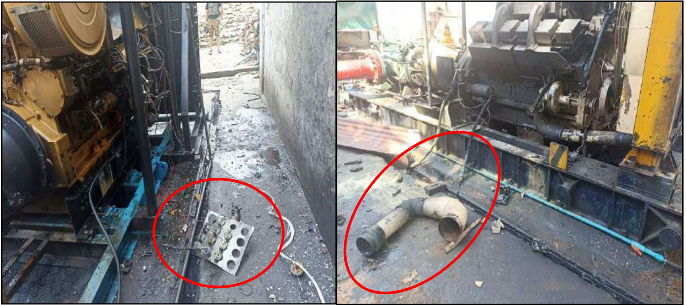
Damages of Water Pump Plant owned by Myanmar Oil and Gas Enterprise in the aftermath of IED attack of PDF terrorists
