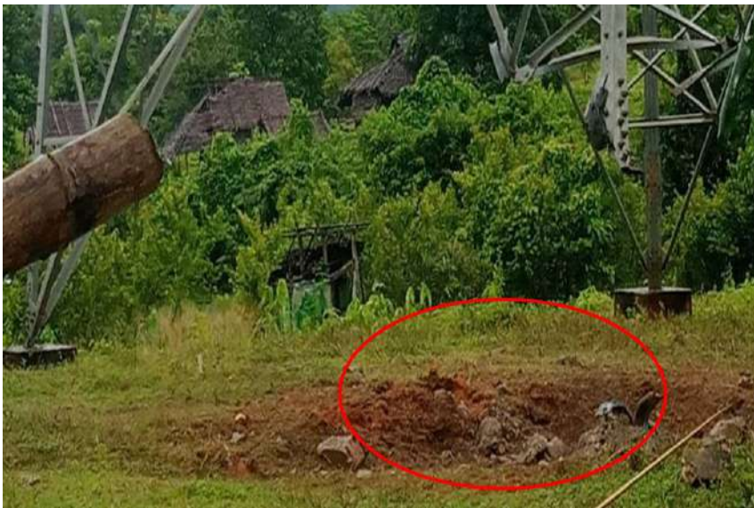
Damages of No. (172) tower in the aftermath of mine attack of KKO (Splinter Group) and PDF terrorists
